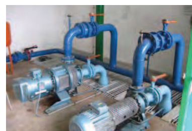
Station de reprise
